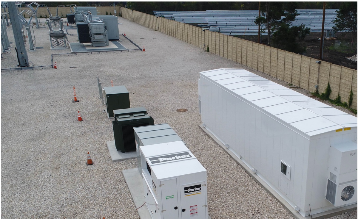
Austin Energy's Kingsbery Energy Storage System is located in a substation and interconnected next to the La Loma Community Solar array.
