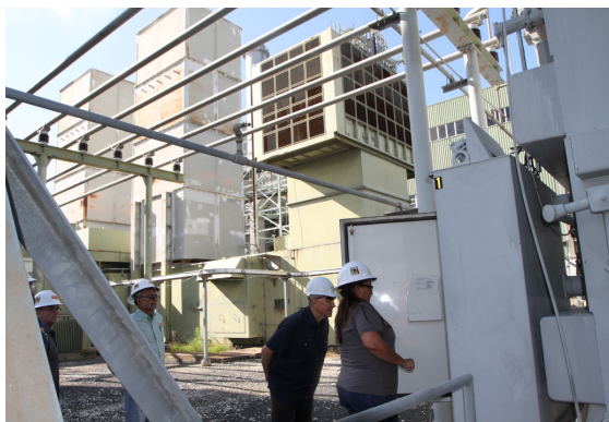
ERCOT inspects Austin Energy peaker units at Decker Creek Power Station.
