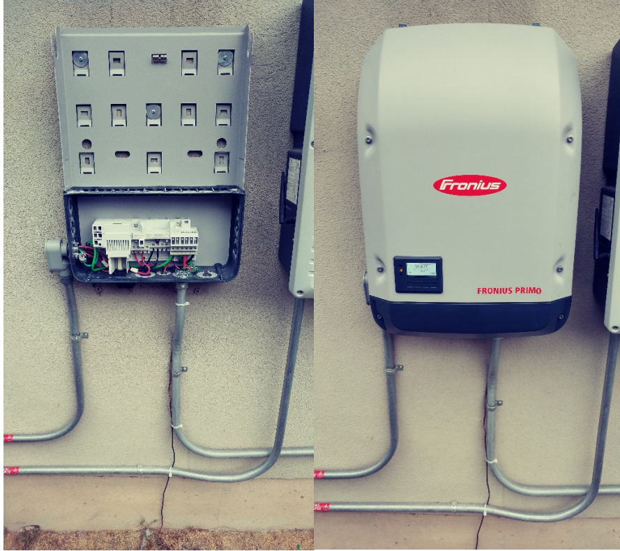
Figure 3-3 Site 19 DUC solar PV control installation (image taken on 3/12/2018)
