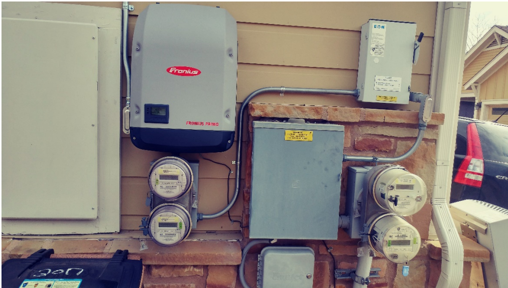
Figure 3-2 Site 14 Autonomous solar PV control installation (image taken on 3/12/2018)
