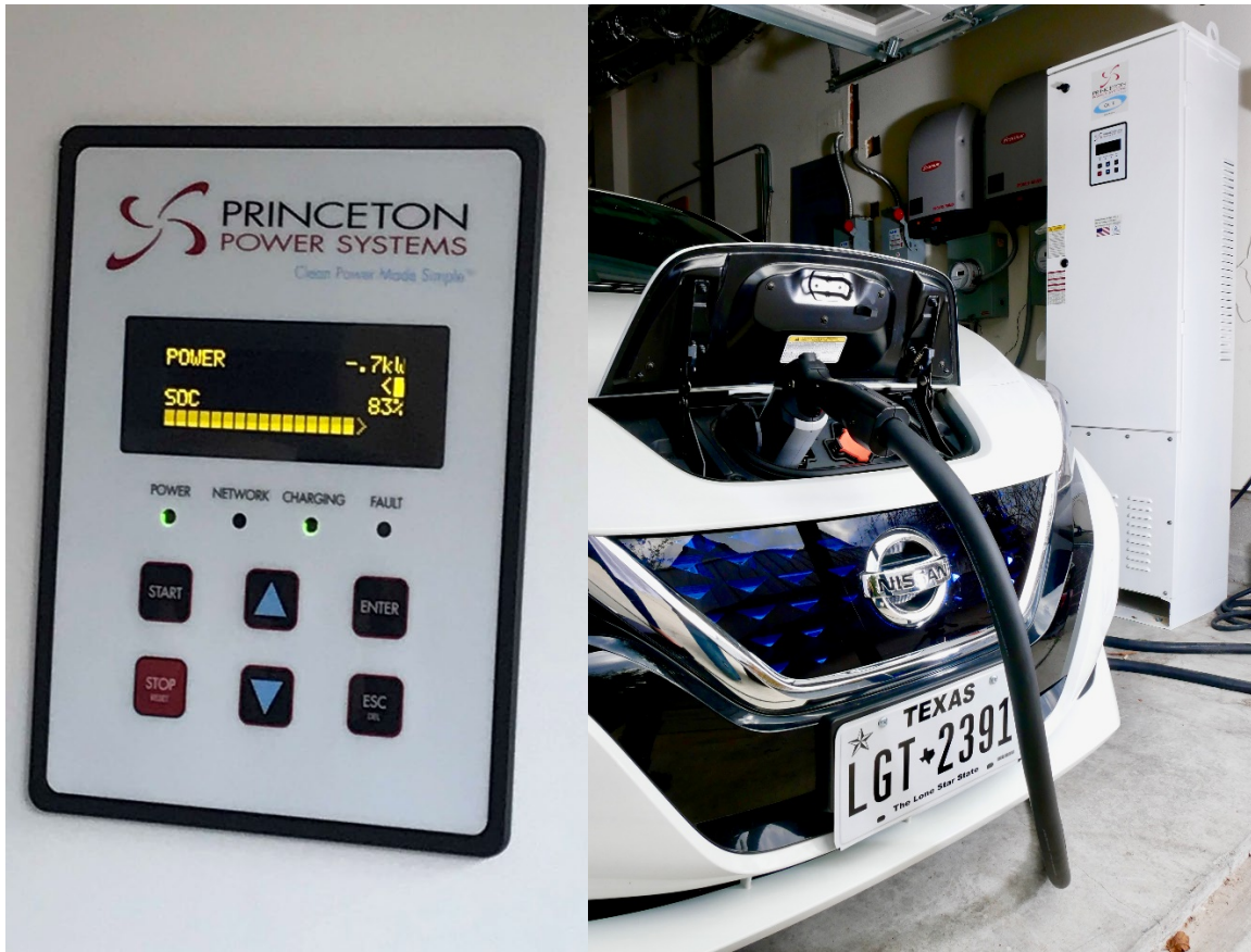
Figure 3-5 Site 25 V2G, Princeton CA-10 Power Systems fast charger (image taken on 11/14/2018)
