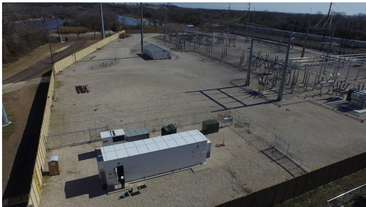
Figure 1-3 KB ESS site view after fencing for substation partitioning installed (image taken on 1/19/2019)
