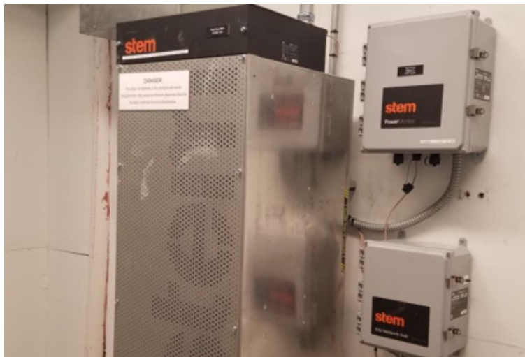
Figure 2-2 Site C ESS installation (image taken on 8/10/2018)
