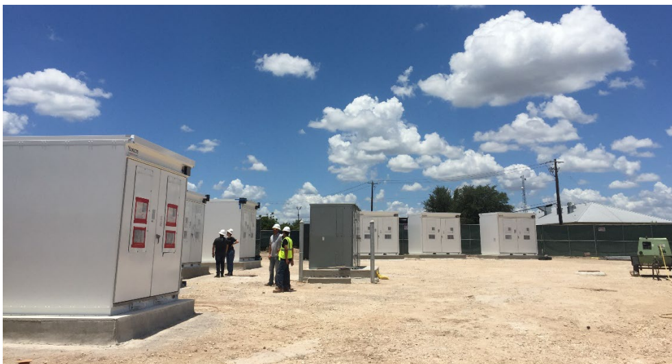
Figure 1-8 Street view of MU ESS battery containers (image taken on 6/25/2018)
