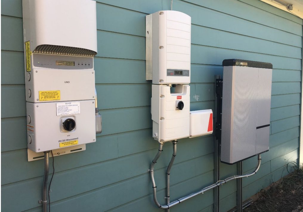
Figure 3-1 Site 2 ESS Aggregated ESS + solar PV control installation (image taken on 1/25/2018)
